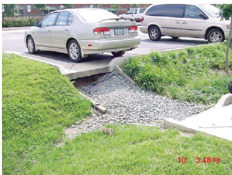
Curb inlets to bioretention swale have eroded because of improper sizing of stone.
