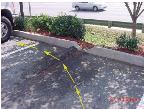
Site runoff by-passes bioretention swale because of small elevation changes during construction.
