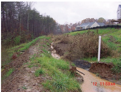
Bioretention swale, installed too early during active construction, has become clogged with sediment.
