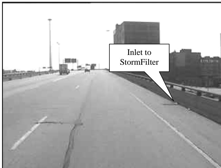
Figure 3-3. StormFilter drainage area condition.
